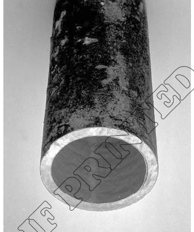
Figure 13 – Minor water damage
